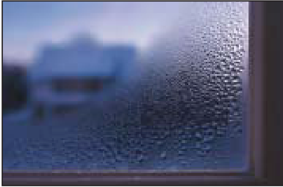
Condensation on the inside of a windowpane.
